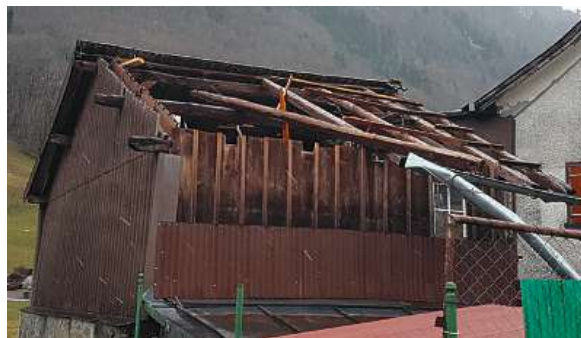
Massiver Sturmschaden in Engi
